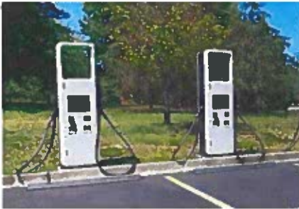
Provide Preferential Parking Spaces for Electric Vehicles
