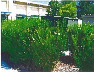
Exterior utility equipment screened with planting
